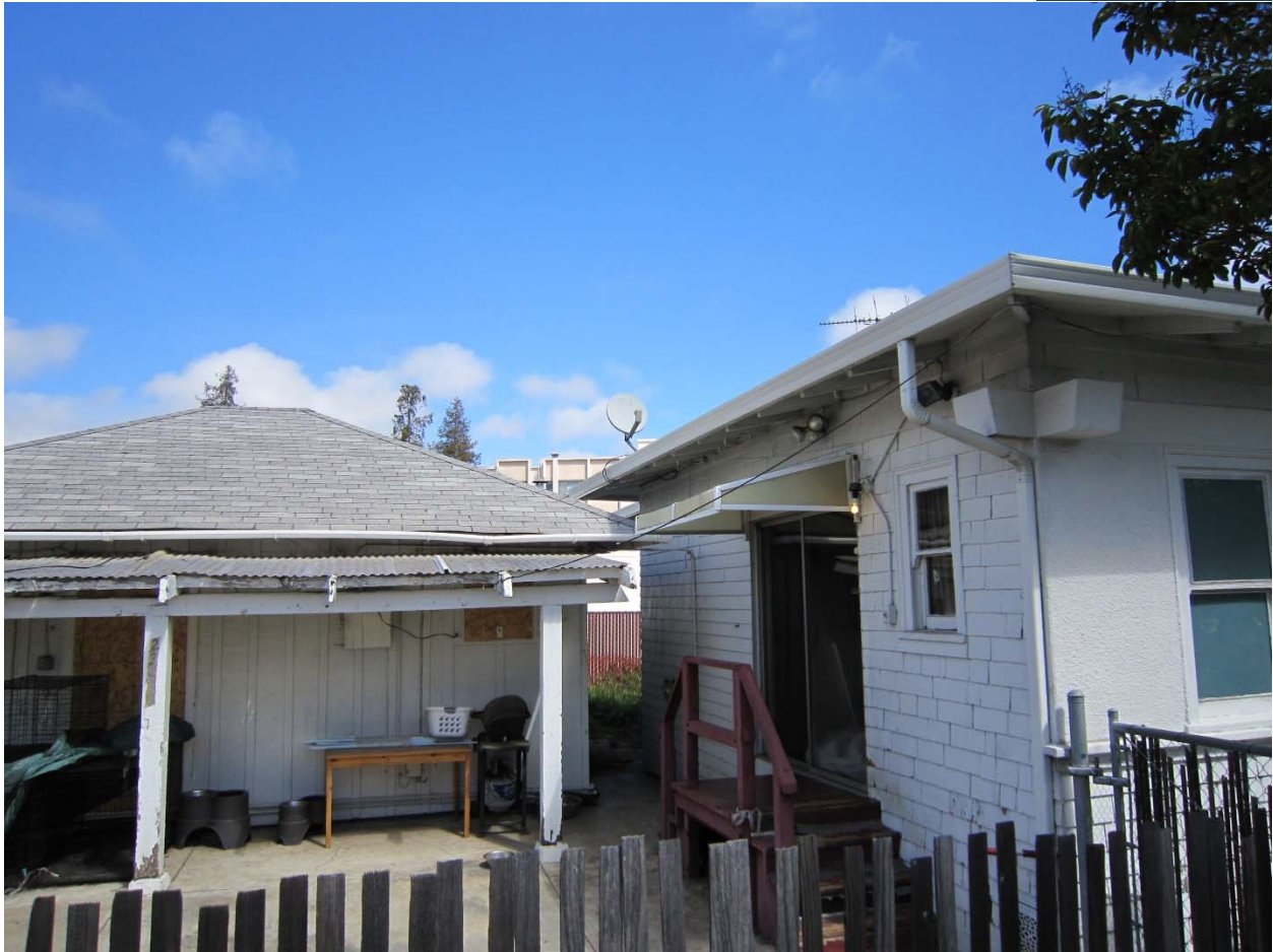
Photograph 4 Property: 22941 Maple Court, Hayward CA View: rear Façade of the house (right), rear porch has been enclosed with a mix of siding materials and an added canopy and stair. A second small building is shown on the left. Date: April 2015
