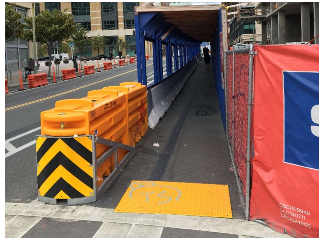
Figure 7. Covered pathway built with detectable, crashworthy channelization devices and detectable warning strip.
