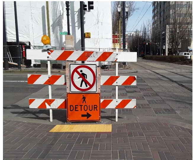
Figure 5. Detectable barrier used in combination with pedestrian detour sign (M4-9b, CA-MUTCD) to denote closed crossing and pedestrian detour.
