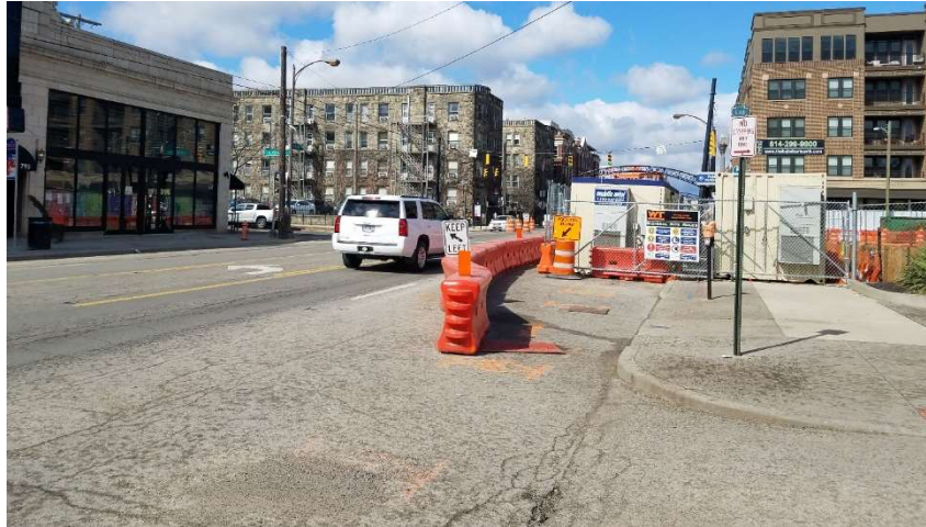
Figure 28. Tapers used to make it clear to drivers that they must stay left to avoid the temporary pedestrian path.
