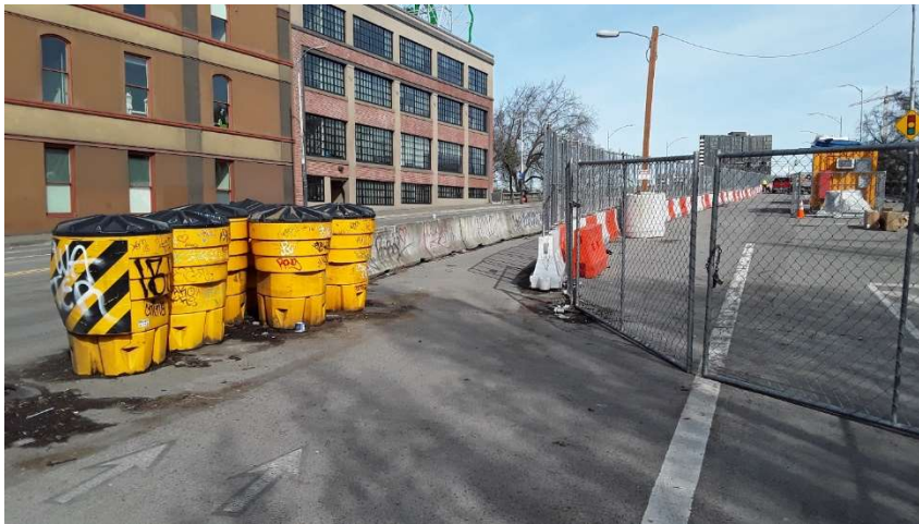
Figure 29. Taper used to direct traffic left to keep drivers out of the temporary multi-use path.
