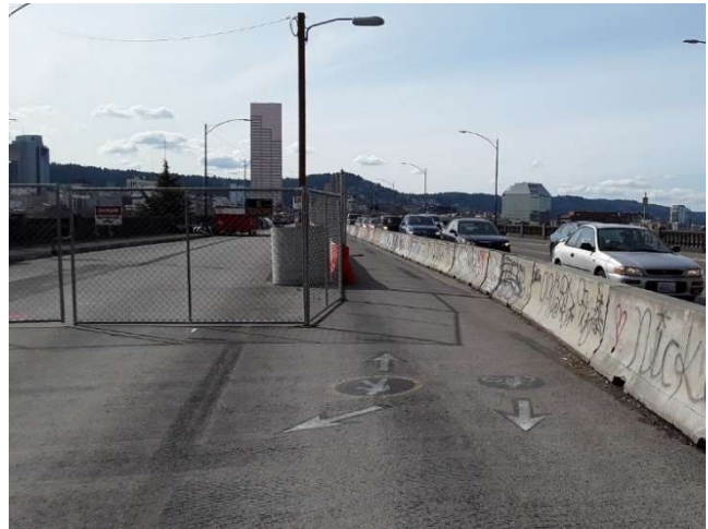
Figure 17. A temporary multi-use path is constructed in a vehicle travel lane to help pedestrians and bicyclists safely cross a bridge when a detour isn't an option.
