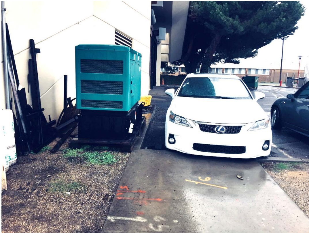
The currently used backup generator with the fuel storage in a belly tank. This is located on the eastern portion of the north side of the Fire Station #6 building.
