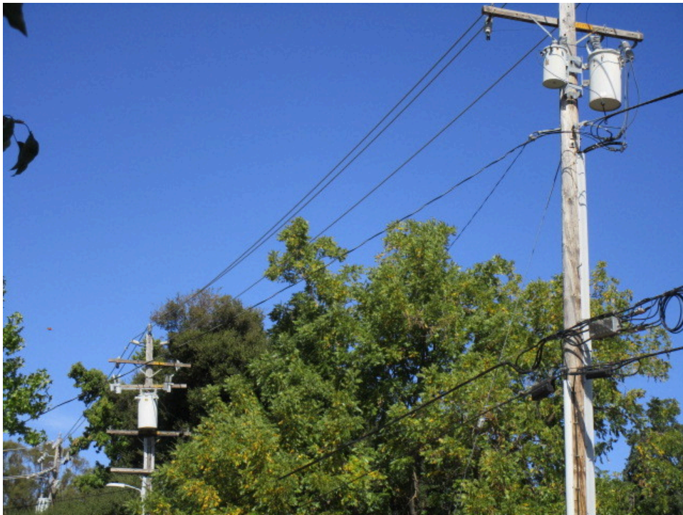
30. Pole-mounted transformers along Rockaway Lane
